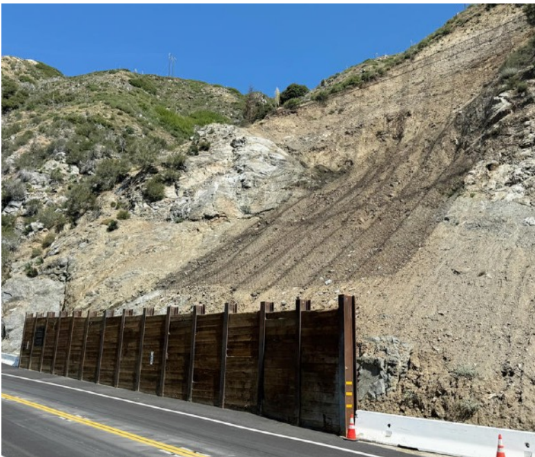
CalTrans repair to ACH between the Red Box/Mt Wilson Rd. and Upper Big Tujunga Canyon Rd. Image Max de Leseleuc
